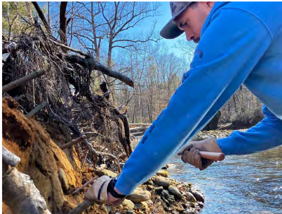
Using live stakes helps speed up natural succession and establish long term ground cover and root systems to prevent further erosion.
